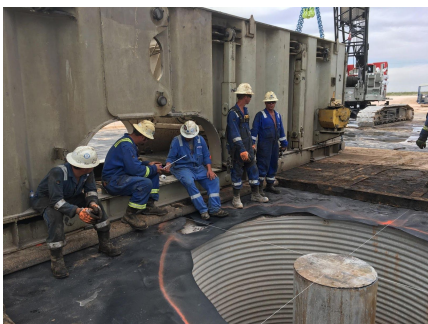
The hole on the ground, before the rig is moved on top of it.
