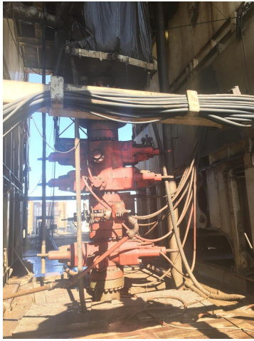
This is called the stack. The stack goes right above the hole. It is a safety measure as it contains multiple ways of stopping gas from coming up. The red wire looking things are hydraulic hoses filled with hydraulic oil. They open and close valves.
