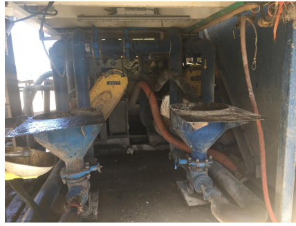
This is where the derrickman mixes chemicals. We pour in sacks of chemicals and pumps bring those chemicals into a mix that contains dozens of barrels of diesel (if we're making oil base). Sometimes we will put in a chemical called bayrite. That will change the thickness of the mix. Sometimes we use calcium chloride. That stuff tingles when you smell it, and it lightly burns your skin.
