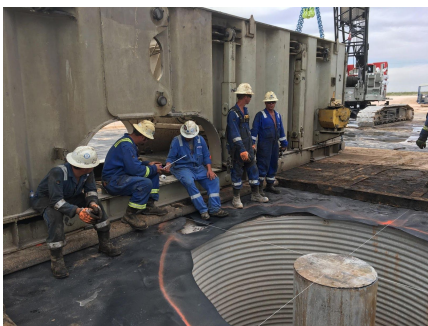
The hole on the ground, before the rig is moved on top of it.
